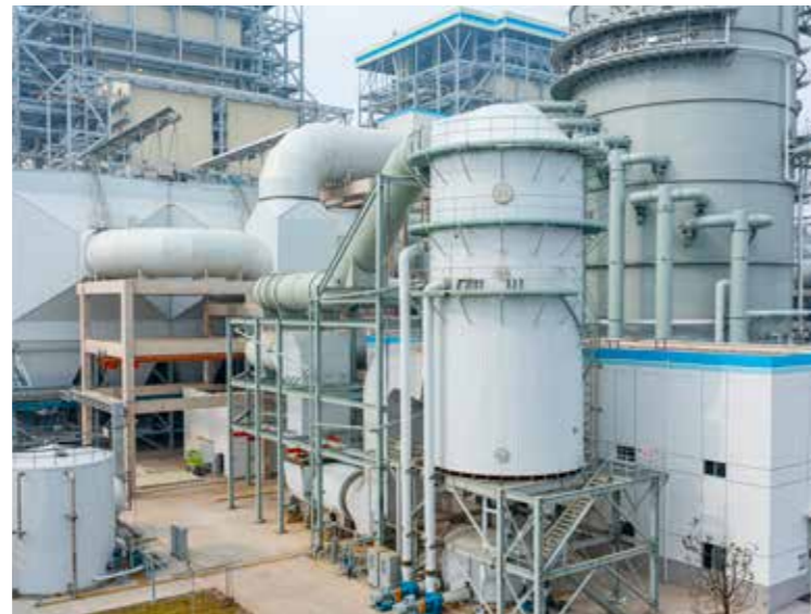
Advanced Desulfurization Wastewater Treatment Plant of Yicheng Power Plant
